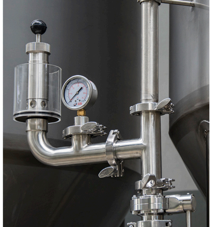
Spunding valve installation
