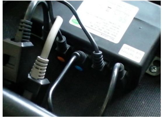
Lifting motor plug connected to control box.
