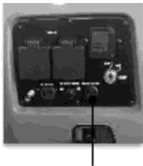
Remote switch 'off' position
