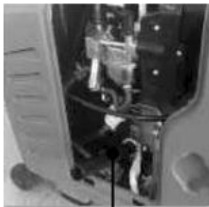
Oil Discharge Pipe
