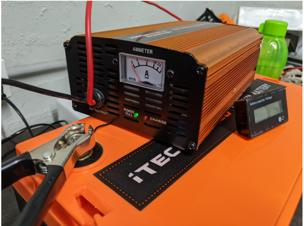
Figure 8 Battery charger connected but not charging
