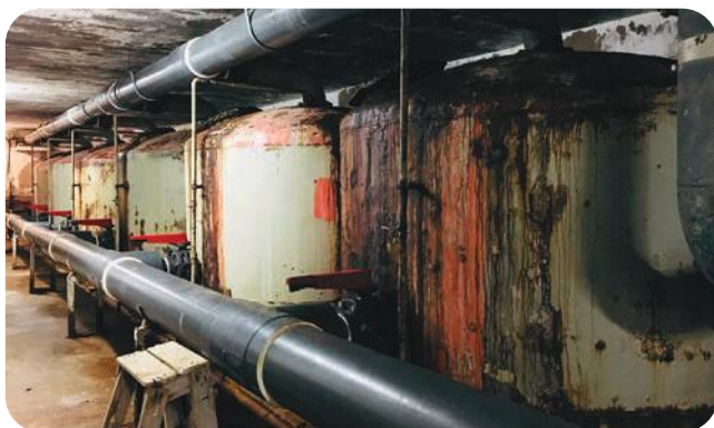
Corroded metal fabricated filters
