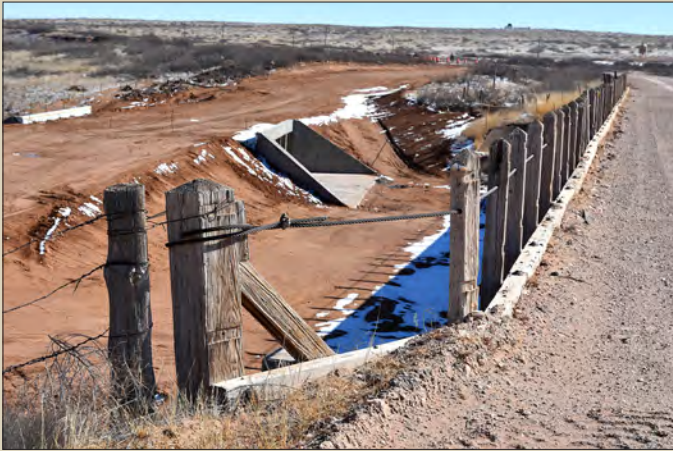
New construction is underway on Dirt 66. Traffic will be forced onto parallel alignments with modern bridges. 1930-era wooden structures eventually will be blocked to all but pedestrians.
