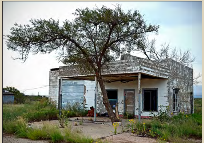
This "Teague Texaco" named after industrial designer Walter Dorwin Teague was a widely-known symbol of the 30s, used in more than 10,000 stations nationwide. This one was left stranded, out of sight and out of luck, when I-40 was built along the northern edge of San Jon. It has since been demolished.
