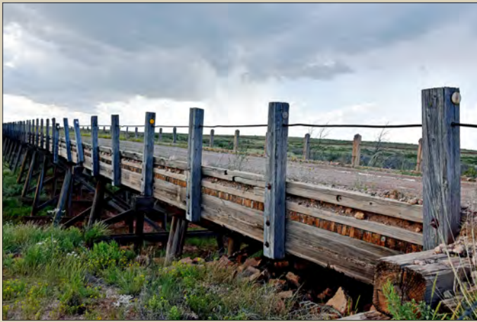
The 1930-era bridges used railroad construction techniques and hardware to connect heavy timbers. The deck has alternating layers much like plywood.
