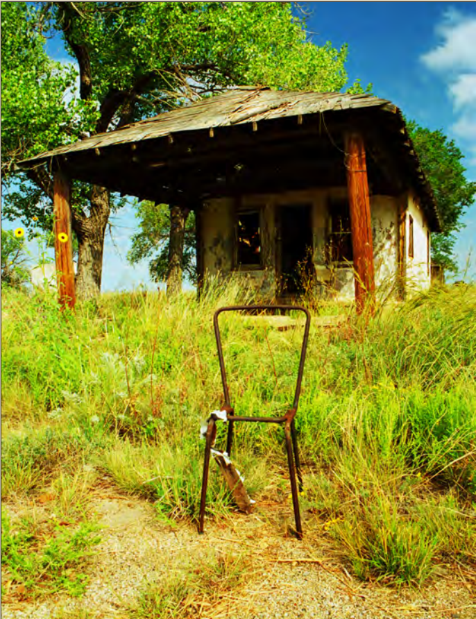
The Broyles Mobil gas station, built around 1925 had a made-from-scratch wooden canopy. It was still intact in this image taken around 2000 but collapsed in this decade. The building has been razed for a marijuana business, legal in NM but not a few feet away in TX.
