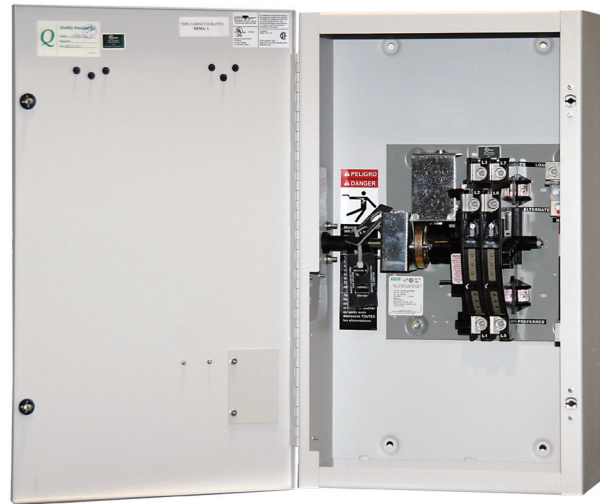
185 Manual Transfer Switch Door Open
