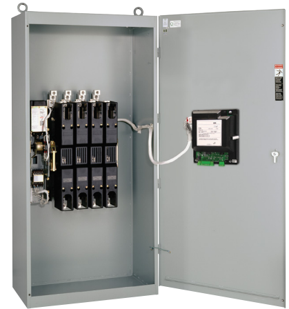
Fig. 5: ASCO Power Transfer Switch rated 1000 Amps
