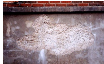
Surface spalling usually associated with freeze-thaw
