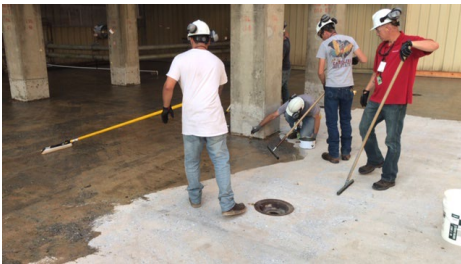
Backroll with ¼” nap rollers; note crewman cutting in around column, he is also brushing out puddles.
