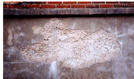
Surface spalling usually associated with freeze-thaw
