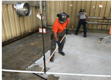
Squeegee- pull tight, no mil buildup, do not allow puddling in cracks and surface gouges.
