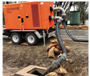
Emergency pump in Barmah.
