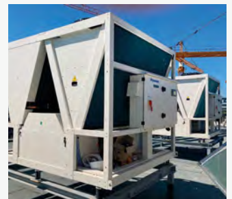
Hungarian Cédrus Liget. A complex facility including apartments, offices and commercial units. Szeged, Hungary. ECOi-W, ECOi and ERV.
