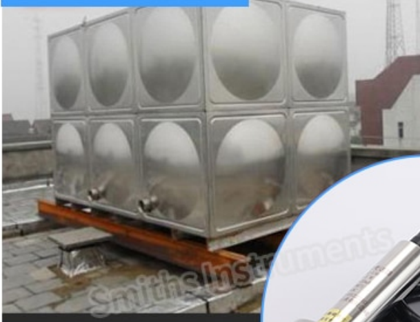
Fire water tank
