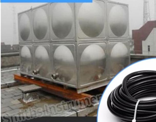
Fire water tank
