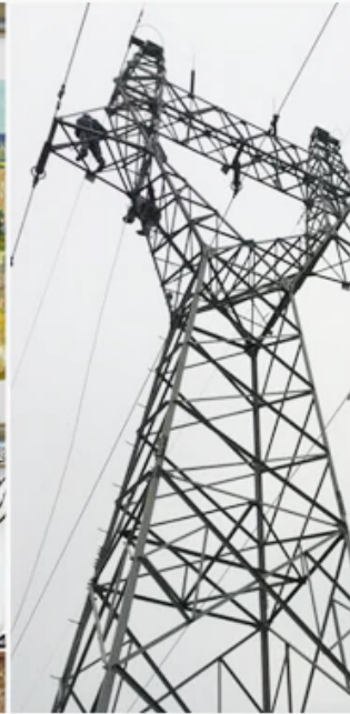
Power grid transformation
