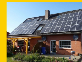
Off-grid home solar system
