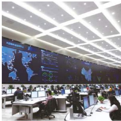
DLP Rear-Projection Cubes or LED Video Wall in Control Rooms
