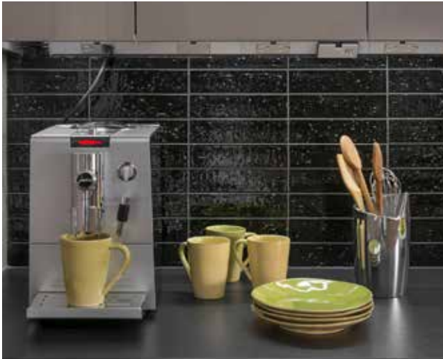
Under-Cabinet Lighting System installed in a kitchen.
