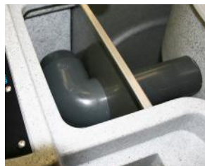
Figure 17.3 - By-pass in operation
