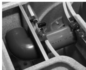
Figure 17.3 - By-pass in operation
