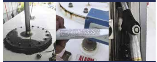
Replace Man Hole Gasket, Faulty Over Fill Alarm, and worn Nozzles
