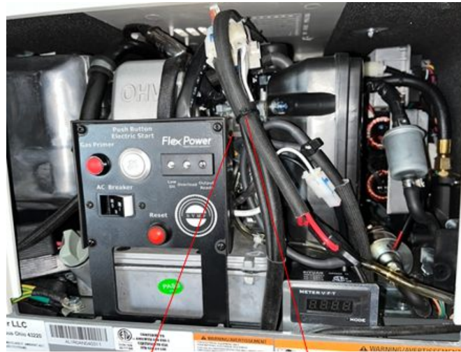
Carburetor (behind this bundle)
