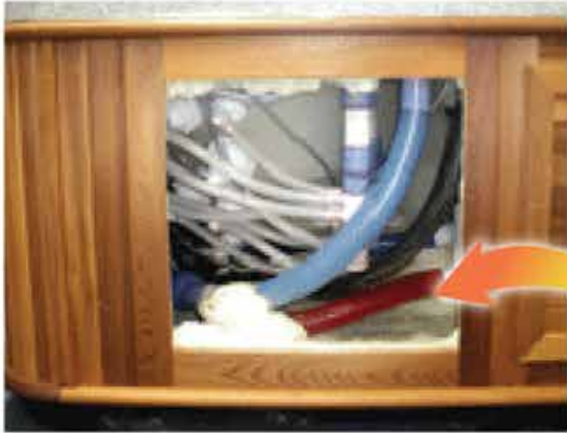
No support for plumbing.
