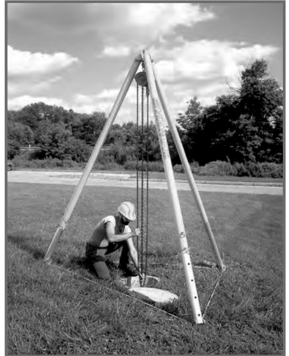
A worker using a Spanco Tripod with Mud Feet to lift a manhole cover single-handedly.
