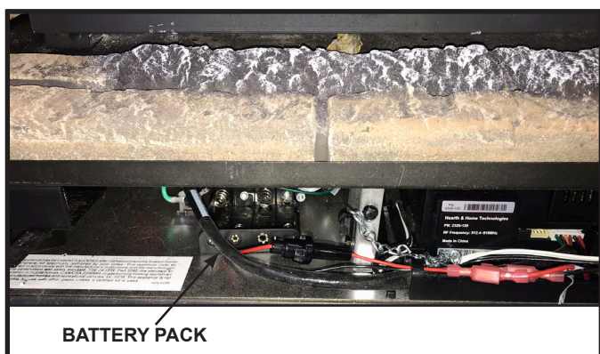
Figure 3.8 Battery Pack Installed
