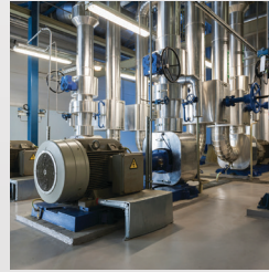
Potable water treatment plants
