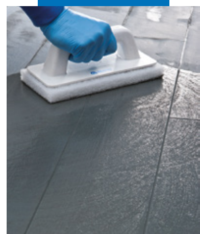
Cleaning the joints with a Scotch-Brite pad (when the product is semi hardened)
