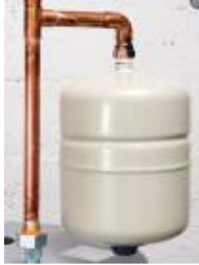
Fig. 5 - A thermal expansion tank helps protect the home's plumbing system from pressure spikes.
