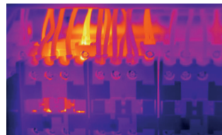
Maintaining plants: Identify excessively high temperatures in circuit breakers and electrical components before breakdowns can occur.
