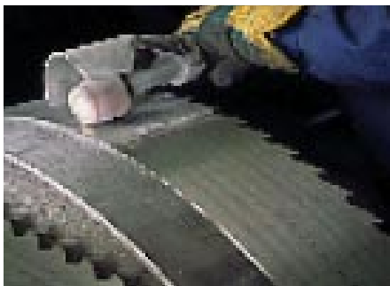
Polishing the weld with a rotary polisher will give the joint a smooth surface.
