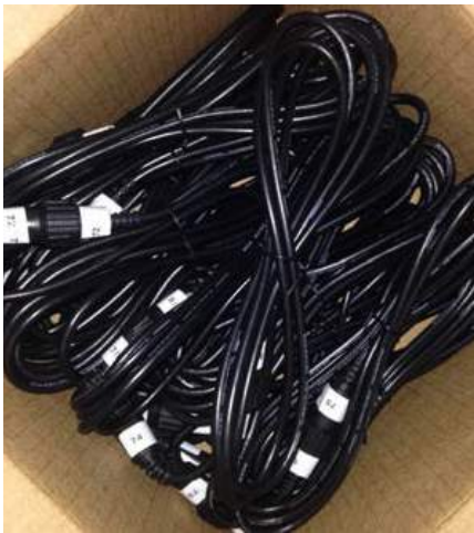
Data Cable Extenders are labeled on each end to match the NDB and the branch
