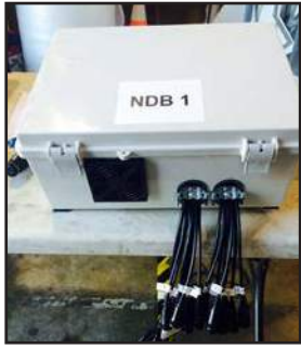
NDB Channels connect to the labeled NDB Data Cable Extenders pictured below
