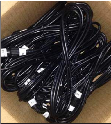
Data Cable Extenders are labeled on each end to match the NDB and the branch
