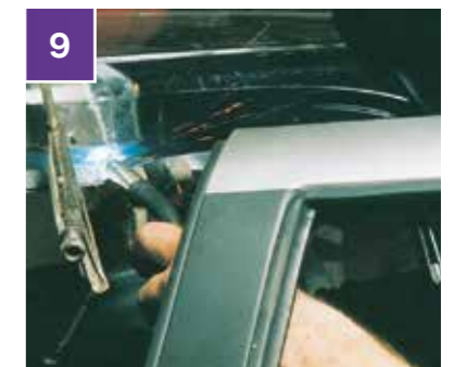
9 Weld appropriate areas. You may weld as soon as panel is fixed with clamps.
