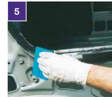
5 Apply primer according to paint company recommendations to repairs, keeping spray area to a minimum and avoiding hard edges. Dry to paint company recommendation.
