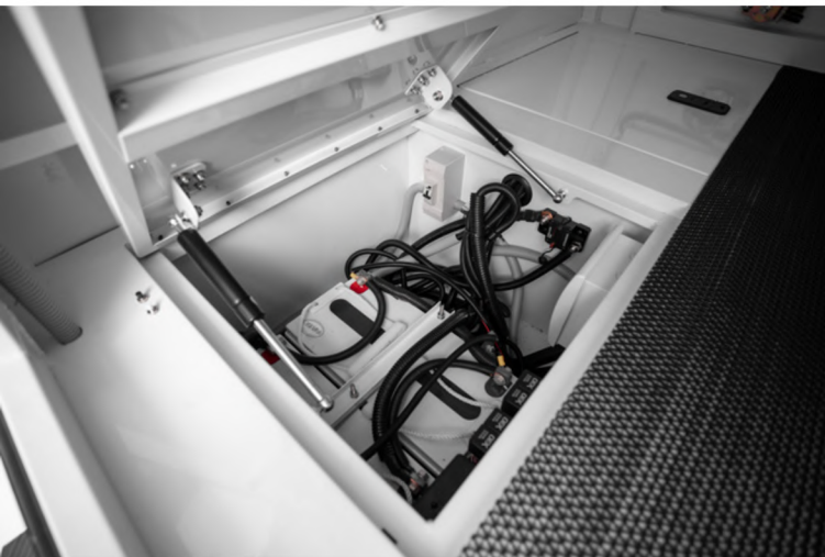
TWO 100AH AGM BATTERIES & 2000W SMART INVERTER
