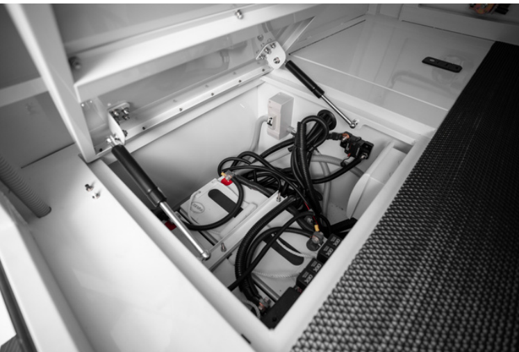
TWO 100AH AGM BATTERIES & 2000W SMART INVERTER
