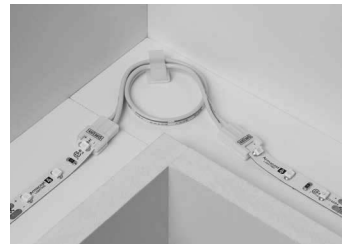
Using a wire lead connector to make a corner turn
