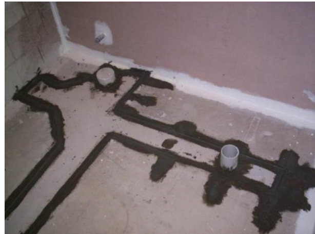
Figure 12 NOVITHOR Cementitious Parge over cold joint between old and new concrete and around pipe penetrations.
