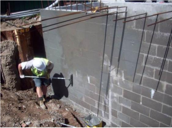
Figure 3 Ensure block work has been wet down with water before applying the first coat of NOVITHOR Cementitious Parge using a soft broom. (This will ensure product penetration and adhesion to block work.)
