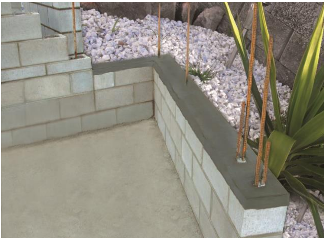
Figure 33 NOVITHOR Cementitious Parge extending 75 mm down RC block wall to create a minimum 75 mm inspection zone.
