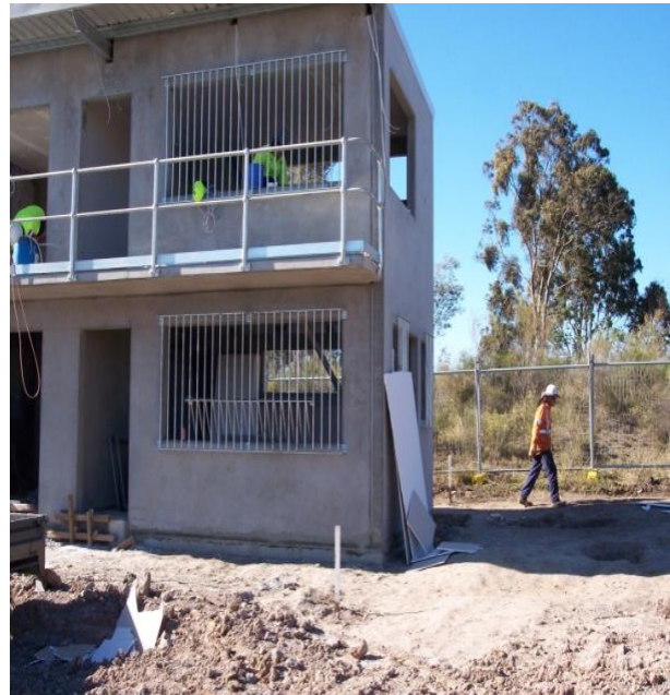
Figure 31 Example of NOVITHOR Cementitious Parge applied as grouting between tilt slab panel and concrete slab.
