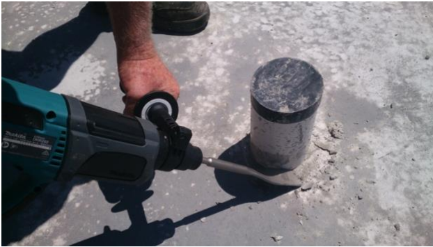
Figure 15 Using a rotary hammer drill with a flat chisel bit, chip out a recess in the slab approx. 5 mm deep.
