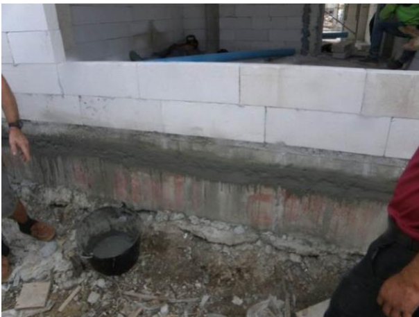
Figure 10 NOVITHOR Cementitious Parge over cold joint between concrete slab and footing plinth.
