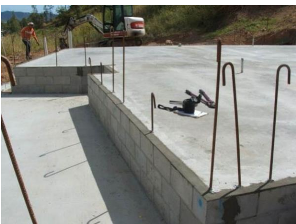
Figure 11 NOVITHOR Cementitious Parge over cold joint between concrete slab and concrete block. Refer page 27.
