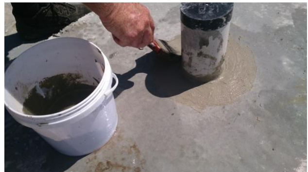
Figure 20 Apply Parge to base of pipe with a soft brush & ensure recess is full with no gaps and extends 50 mm.
