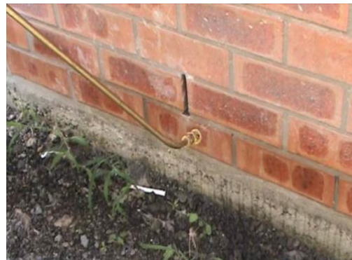
Figure 39 Applied to face bricks work. 1 st coat focus on mortar joints; 2 nd coat cover brick face to blend any runs.
