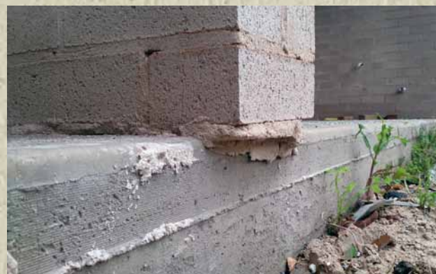
Overhanging brickwork with mortar fill correctly applied to the outside core holes.
