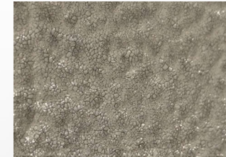
Poor coating film
