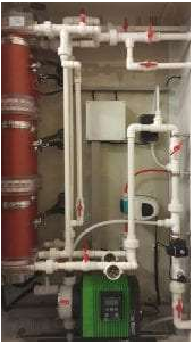
ELA-20 000 interior of the hydraulics
