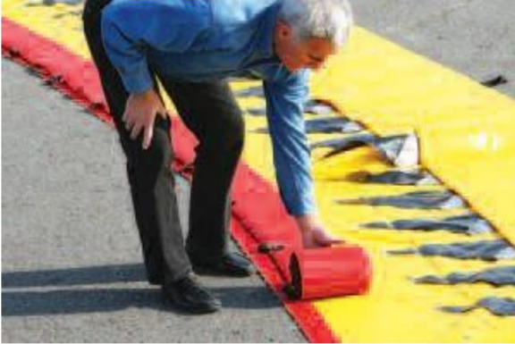
3 – Add a second ballast over the entire length to avoid water infiltration.
