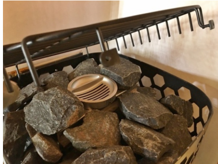
BWT tank, tank lid, and the vent cover installed and the rocks placed around the tank.
