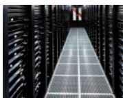
Telecom base station
