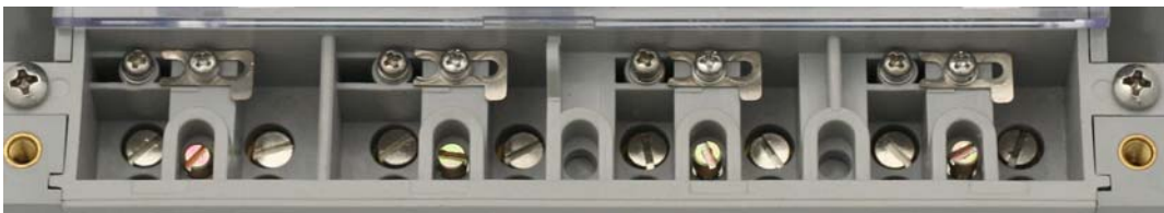
• Figure 6-9 Meter with the CT to VT links disconnected by sliding shims.
