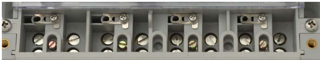
• Figure 6-10 Meter with the CT to VT links disconnected by removing screws.
