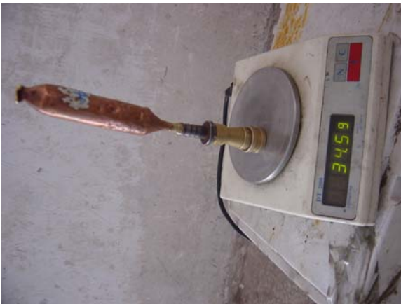
4-7-16、 Connect the canned bottle with the process tube and then compressor work for more than 5 minutes, charge the refrigerant into compressor
