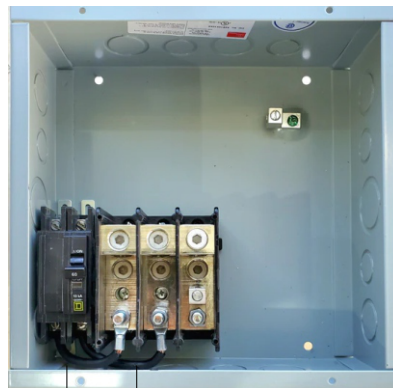
Splicing Hardware EV Charger Breaker
