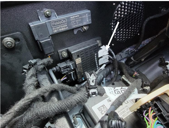
Plug modules back in that had been relocated to side of the console.
