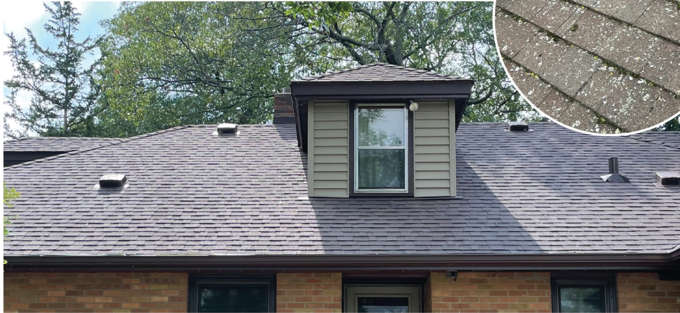
Typical dark asphalt shingle surface temperatures range from 140°– 168°.
