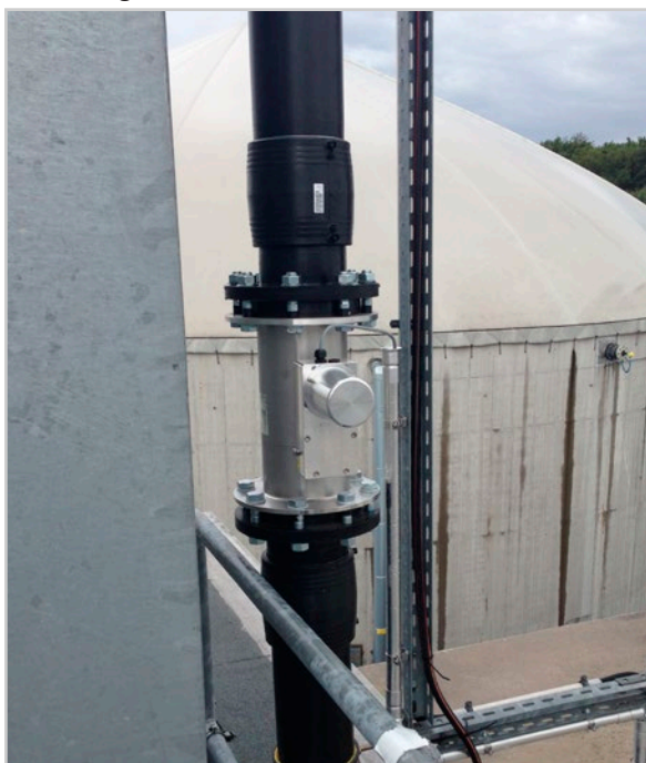
Installation of the GD 300 (Ex) in a vertically falling pipeline
